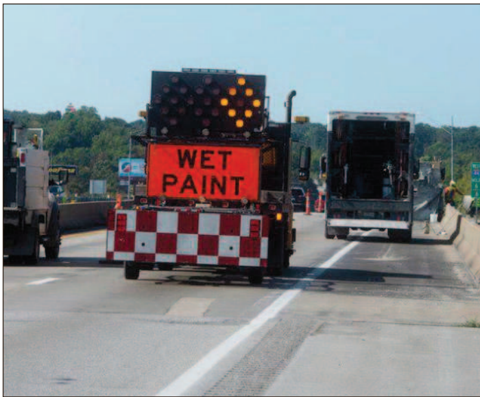
Missouri Department of Transportation workers repaired a bridge on Interstate 44 over Main Street in Joplin in 2020. A chunk of the bridge decking had broken loose and opened a hole in the I-44 bridge.
